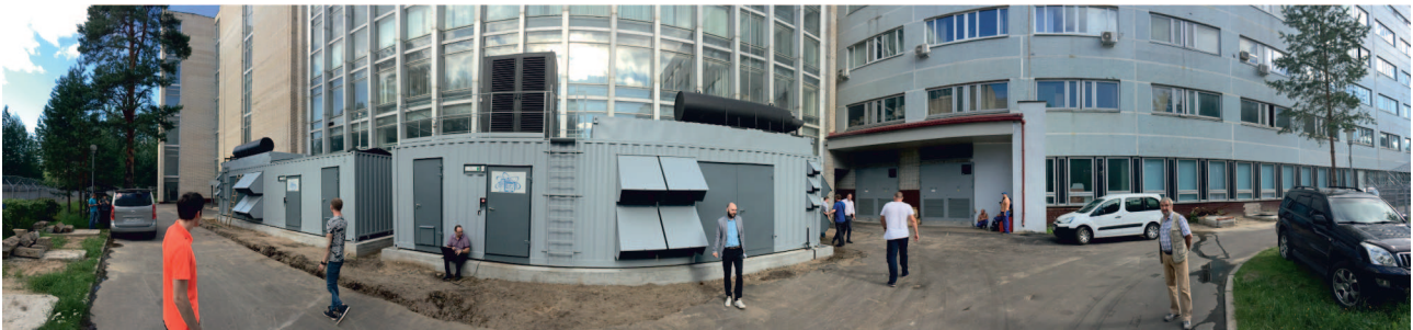
Figure 8. Diesel generator units near MLIT.
