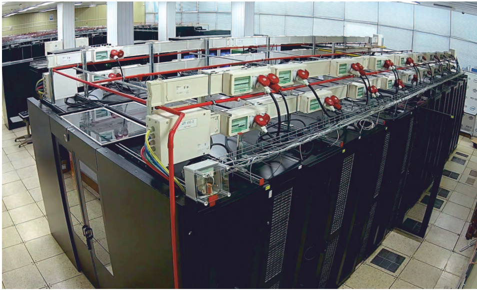
Figure 5. Module 4 using the cooling of the cold corridor of the module with inter-row air conditioners.
